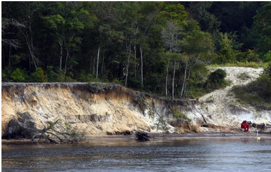
Figure A7.4 - Northern bank, 300 m to the east of the new bridge. Access for fishing does not help but is not a primary source of erosion.
