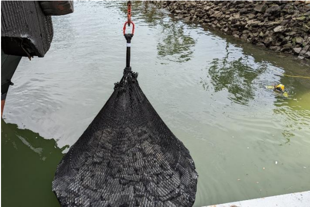
Figure 8: Photo of a large rock bag being craned into position with a diver on standby
